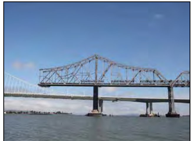
The existing East Span Cantilever Section of the San Francisco-Oakland Bay Bridge Being Dismantled
