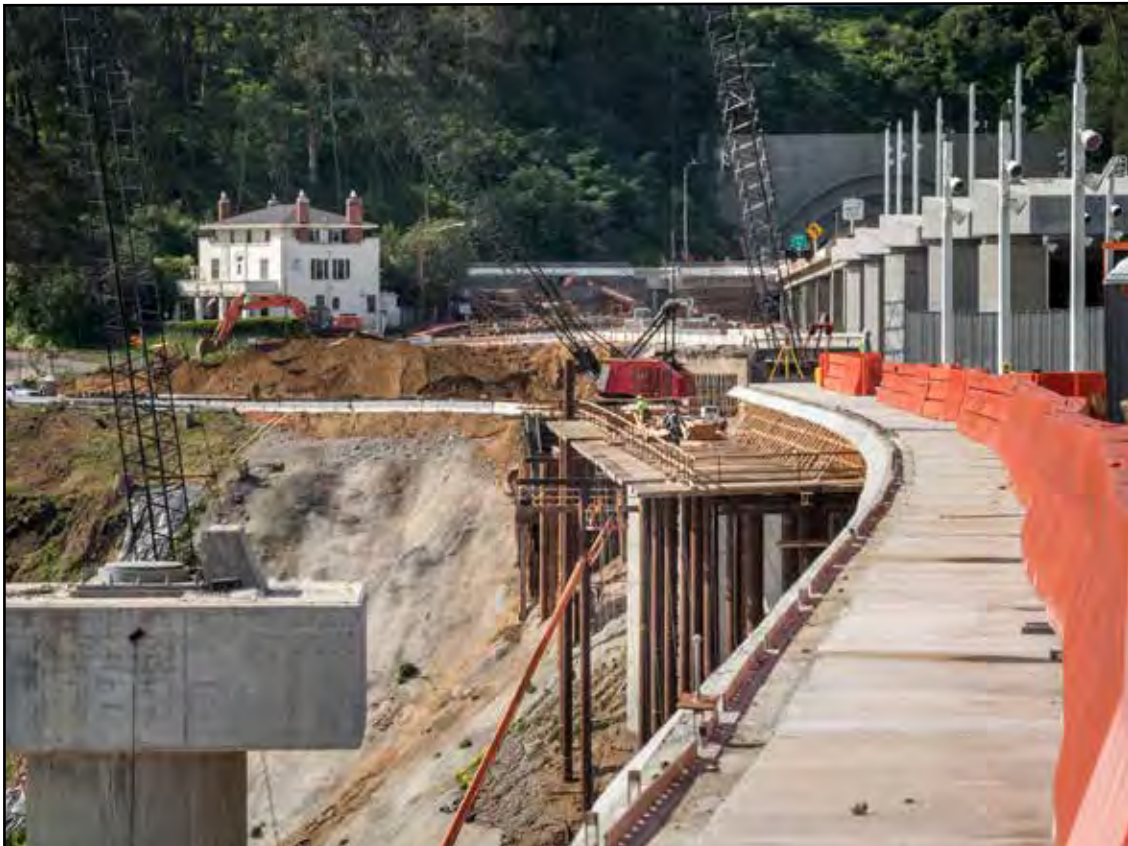
Eastern Span of the San Francisco-Oakland Bay Bridge Bicycle/Pedestrian Path Construction in Progress
