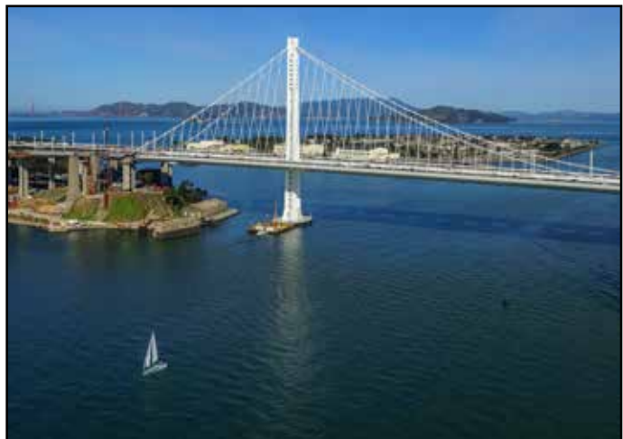
Aerial View of New Bridge as Old Bridge Continues to be dismantled
