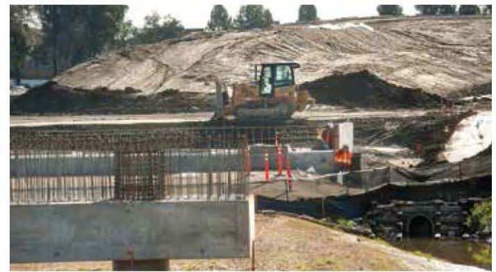
BART to Silicon Valley is a major project in Plan Bay Area. Pictured above is a rendering of the Berryessa Station and the extension's construction (Photo: Noah Berger).
