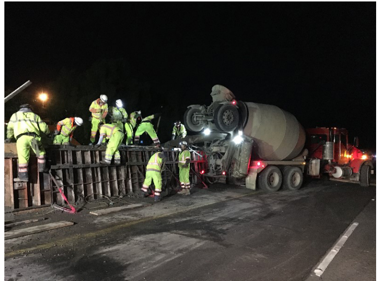
Construction crews working on a concrete pour for the median barrier replacement.
