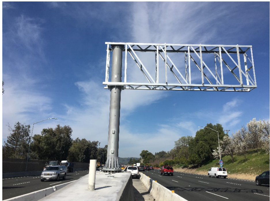
An overhead sign frame that will display tolling information. (See additional construction photographs on pages 15-17)
