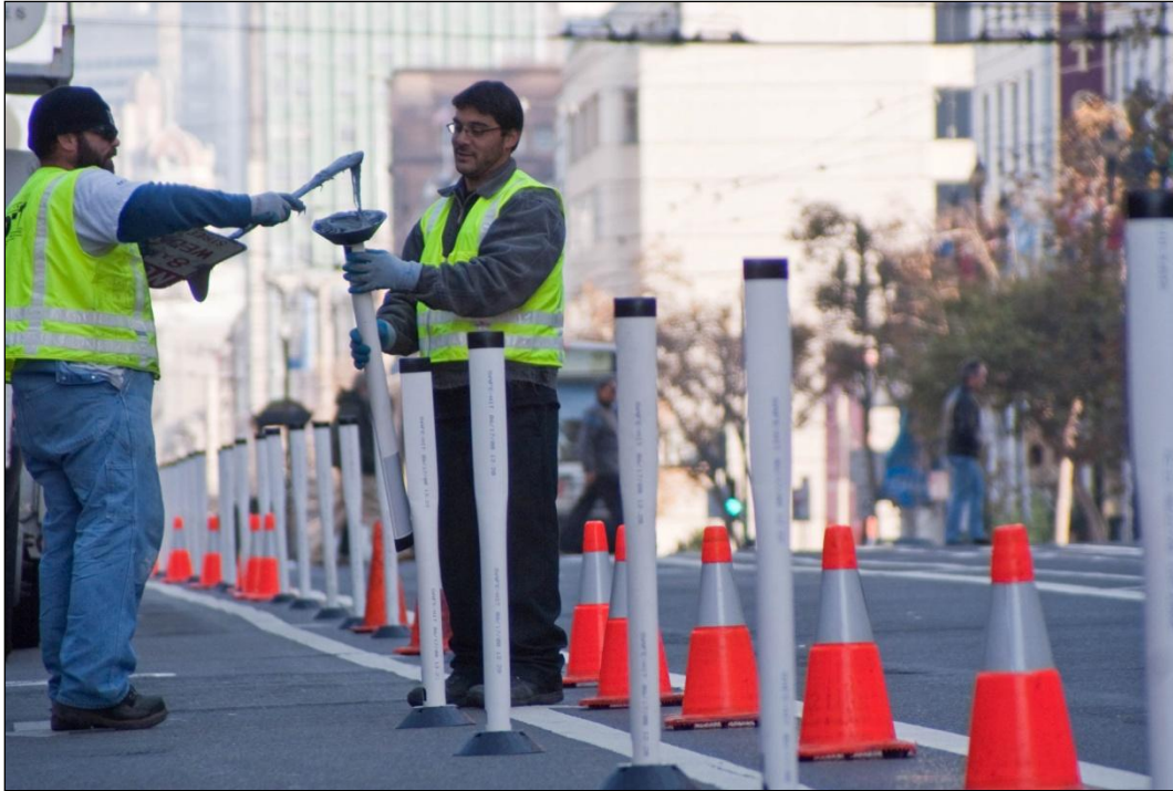
Figure A3-8 Safe-Hit Posts
