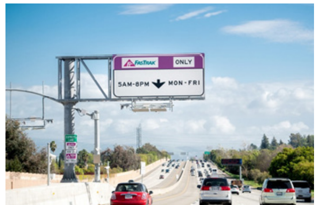
Overhead hours of operation sign and toll system equipment on the I-680 Express Lanes
