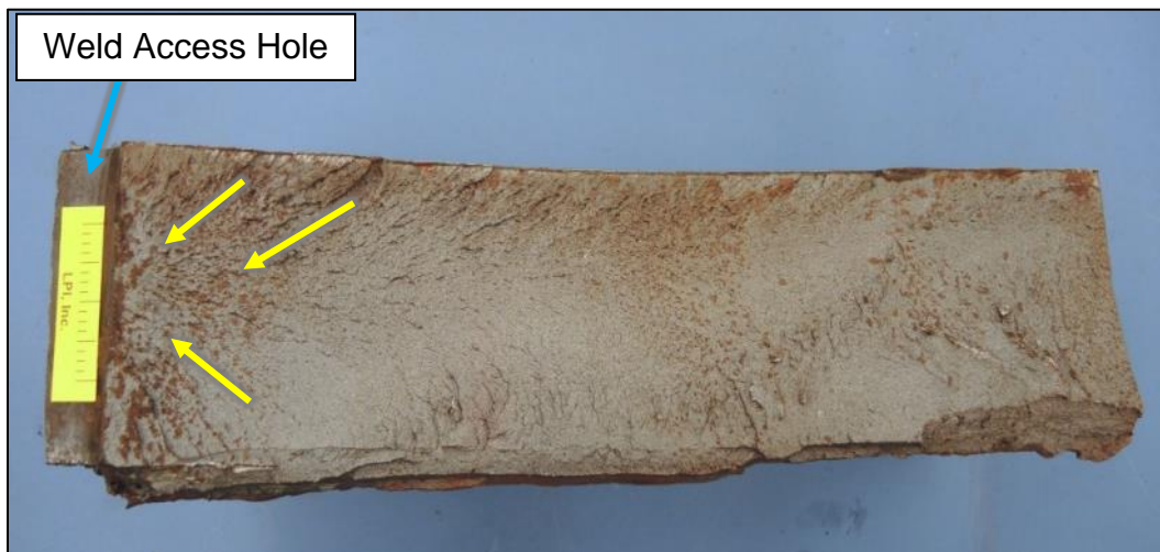
Fig. 10. Chevron marks (yellow arrows) on the fracture surface of girder sample D.4-SW pointing towards the origin at the edge of the weld access hole.
