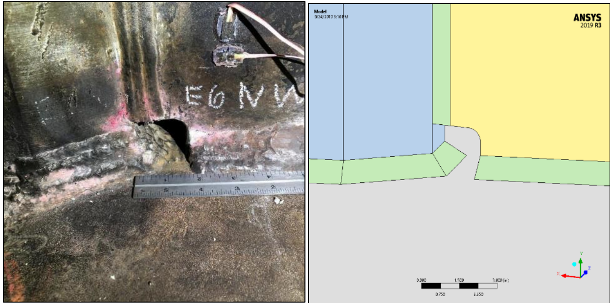
Fig. 143. First Street South (“F”) wrapped fillet welds between bottom flange and hanger (top side of bottom flange).
