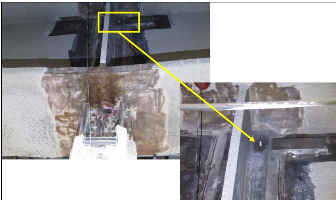
Fig. 188. Typical removal location for the 3-in. diameter core samples removed from girder hangers above Fremont Street and First Street.
