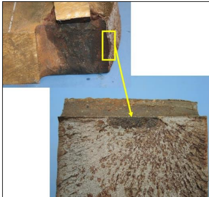
Fig. 13. Dark oxide covered elliptical pop-in crack fracture origin at the weld access hole (top) of girder sample E.6-SW.
