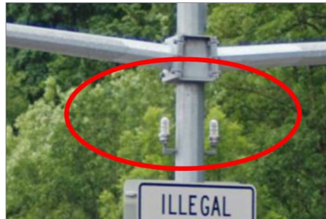
Lights indicate transponder status. Source: WSDOT
