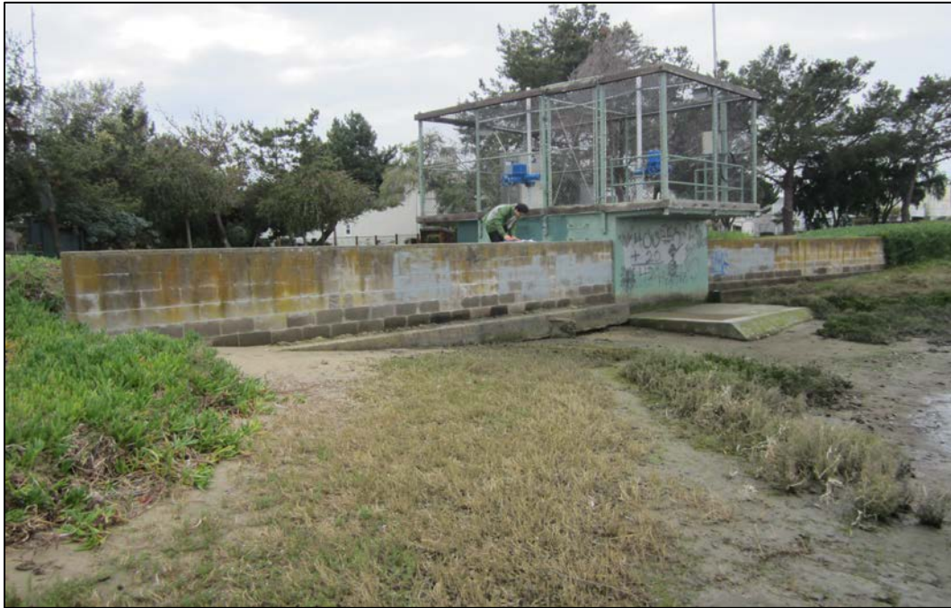
Figure 4. Site A – Tide Gate Structure west of the Doolittle Road/Bay Farm Island Bridge
