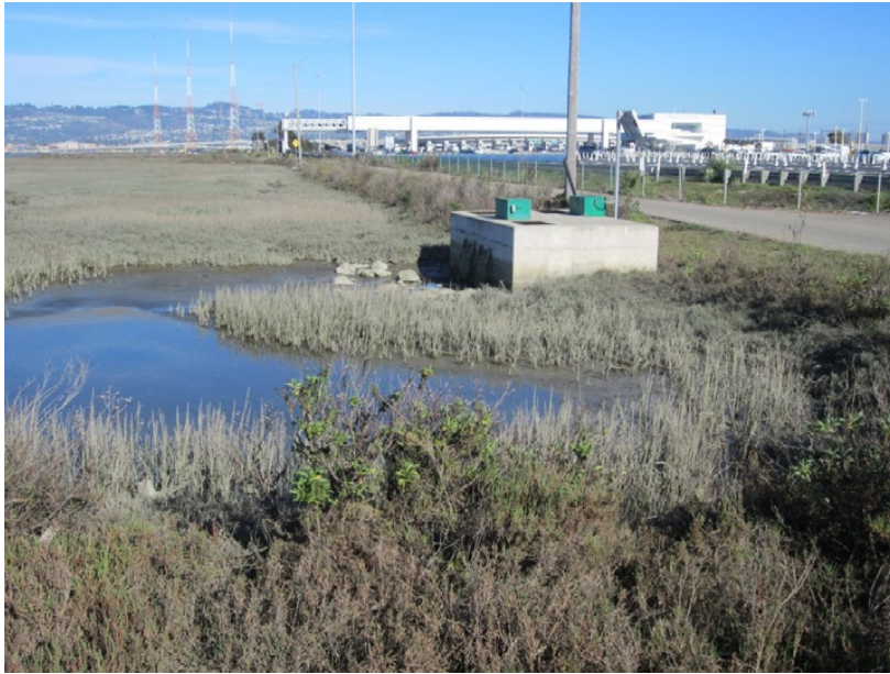
Figure 5-12: A site photo (looking east) of the dirt access road adjacent to I-80. One of many drainage structures owned and operated by Caltrans, can be seen adjacent to the road
