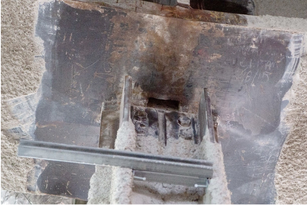
Figure 16 – South Girder – North Half - View Looking South – No Fracture (Photo: TJPA)
