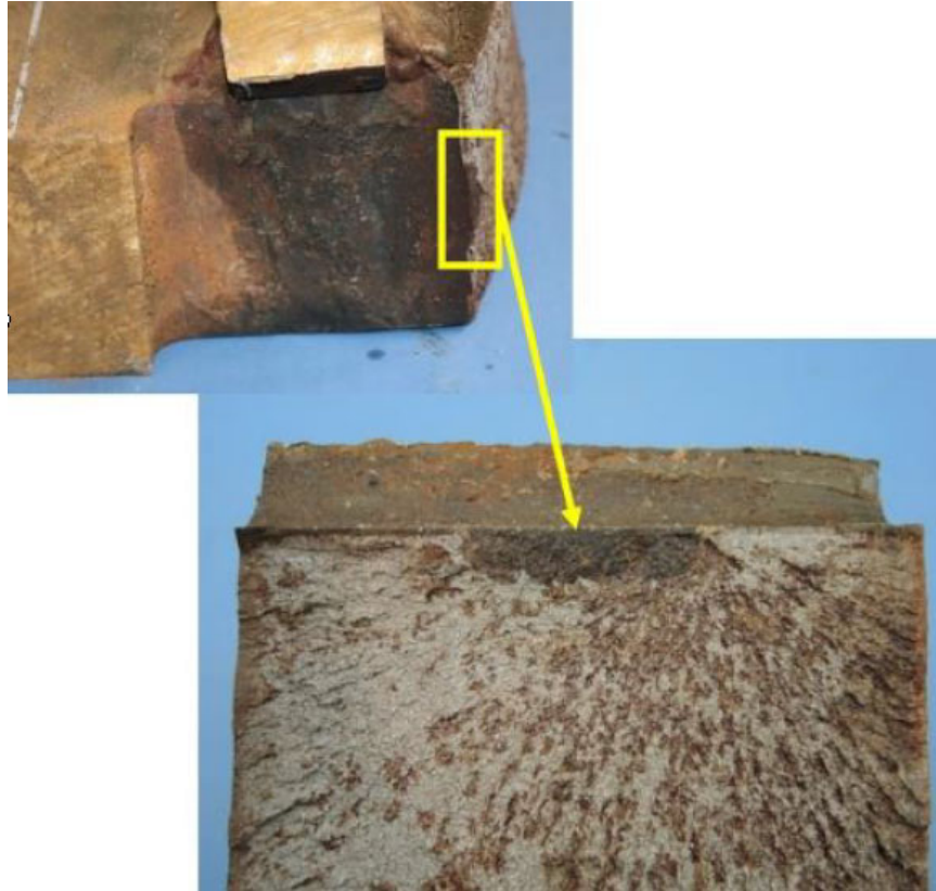
Figure 20 – Pop-in Crack (covered by dark oxide) near Mid-depth of Bottom Flange at South Half of South Girder (Photo: LPI Report)
