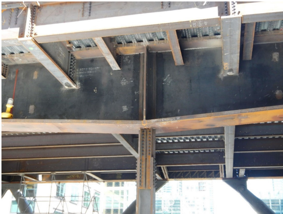
Figure 5 – Photo of a TPG3 Girder during Construction of the TTC (Photo: TJPA)
