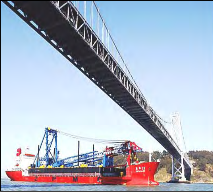
Ship Carrying the Shear-leg Crane Barge Crossing beneath the West Span of the Bay Bridge
