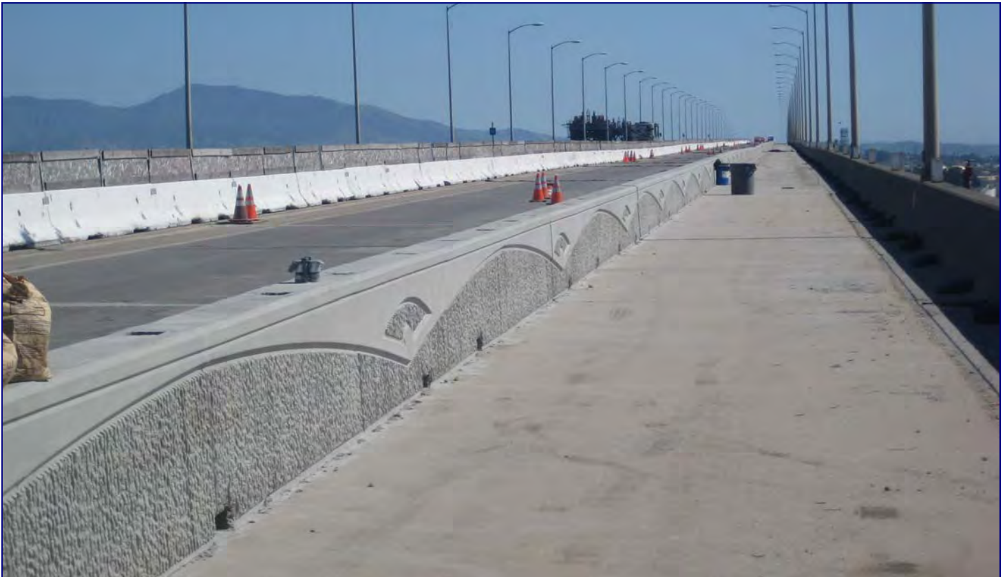
New Pedestrian/Bicycle Pathway Is under Construction on the West Side of the Existing Bridge
