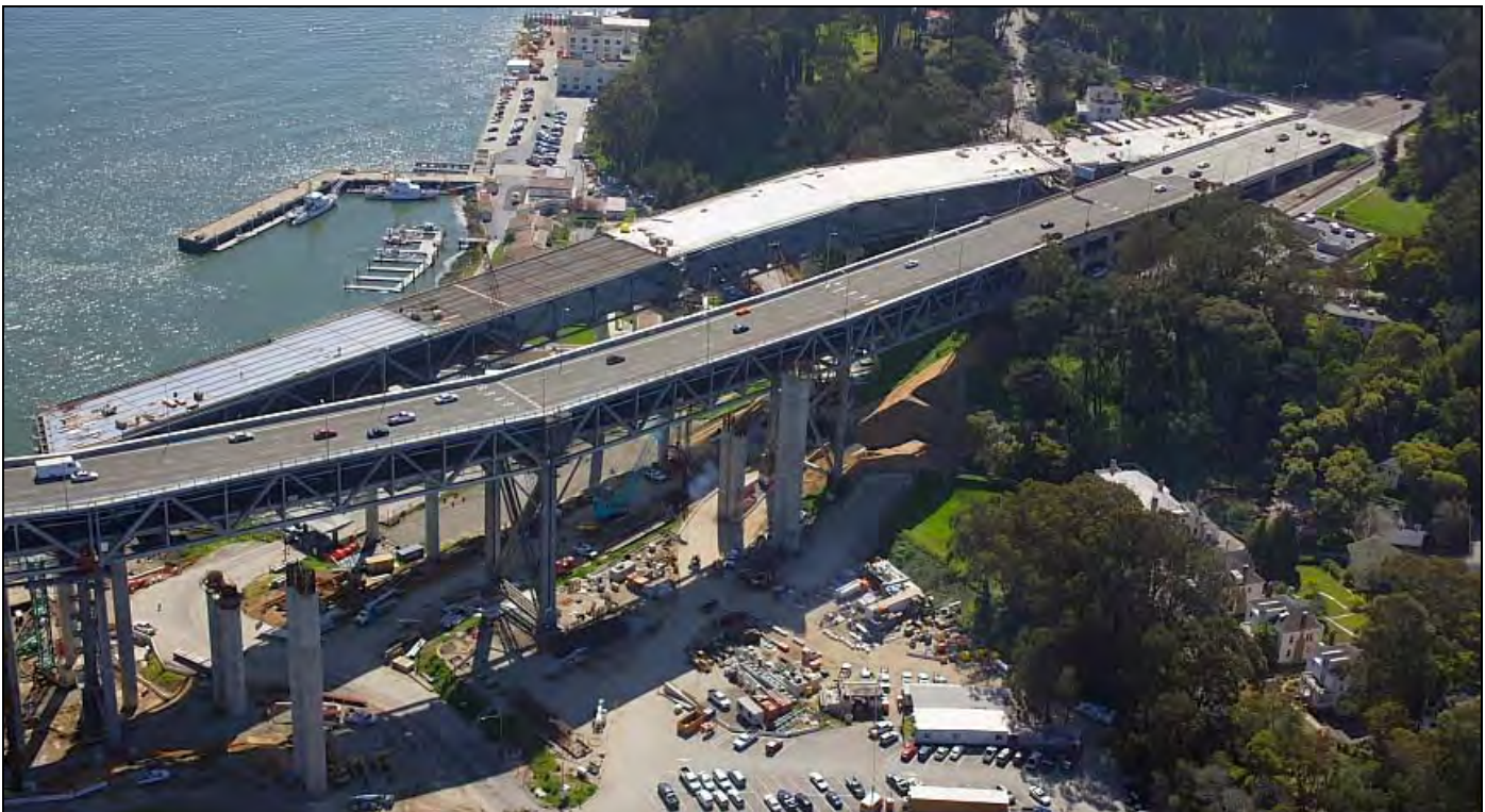
YBITS Advanced Foundation and Column Work Just North Of Existing Viaduct (foreground)
