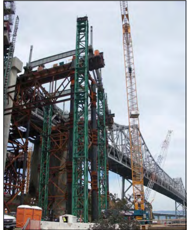
Skid Beams for Roll-Out and Roll-In of East Tie-in Structure under Construction
