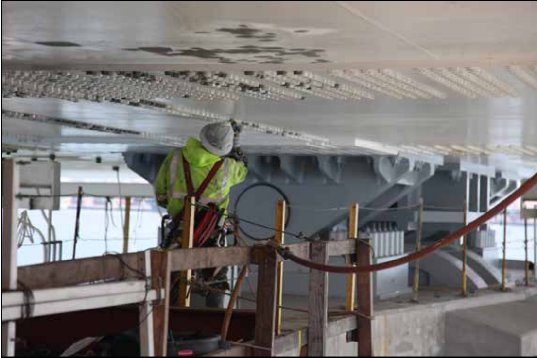
A View of the west Face of Pier E2W with S1 Shear Key Hold Down Retrofit Complete
