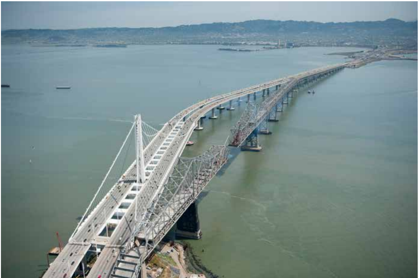
Eastern Span of the San Francisco-Oakland Bay Bridge on Left and Demolition Progress of the Old Bay Bridge on the right
