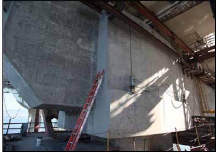
A View of the west Face of Pier E2W with S1 Shear Key Hold-Down Retrofit Complete
