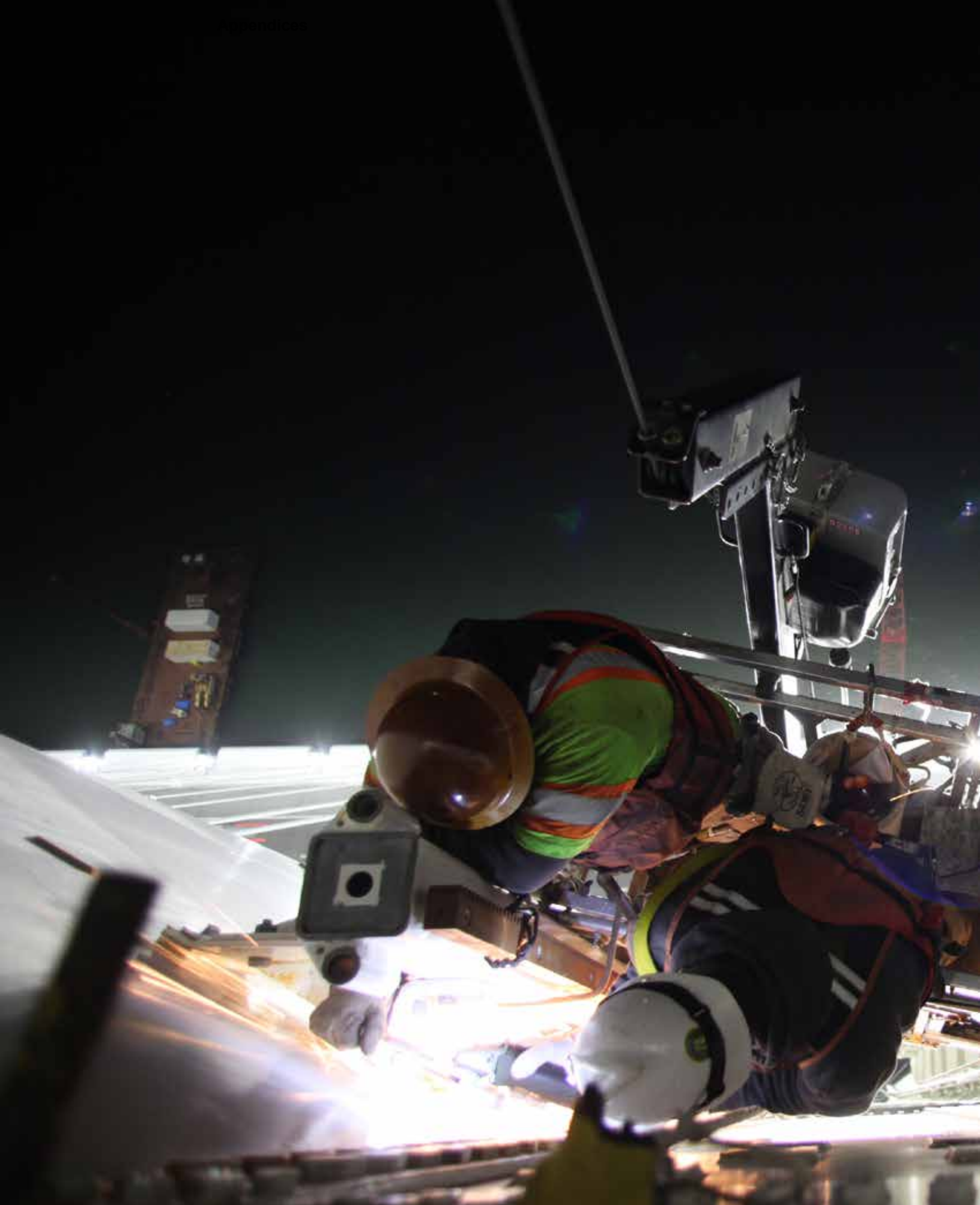
San Francisco-Oakland Bay Bridge Grinding Huck Bolts on the Self-Anchored Suspension Bridge Tower
