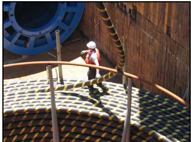
Cable for the Oakland Touchdown Submarine cable project
