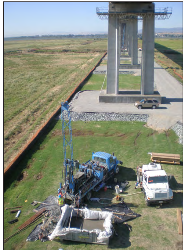
Down Holes Being Drilled for Seismic Monitoring Devices up to 250 Feet Below Grade
