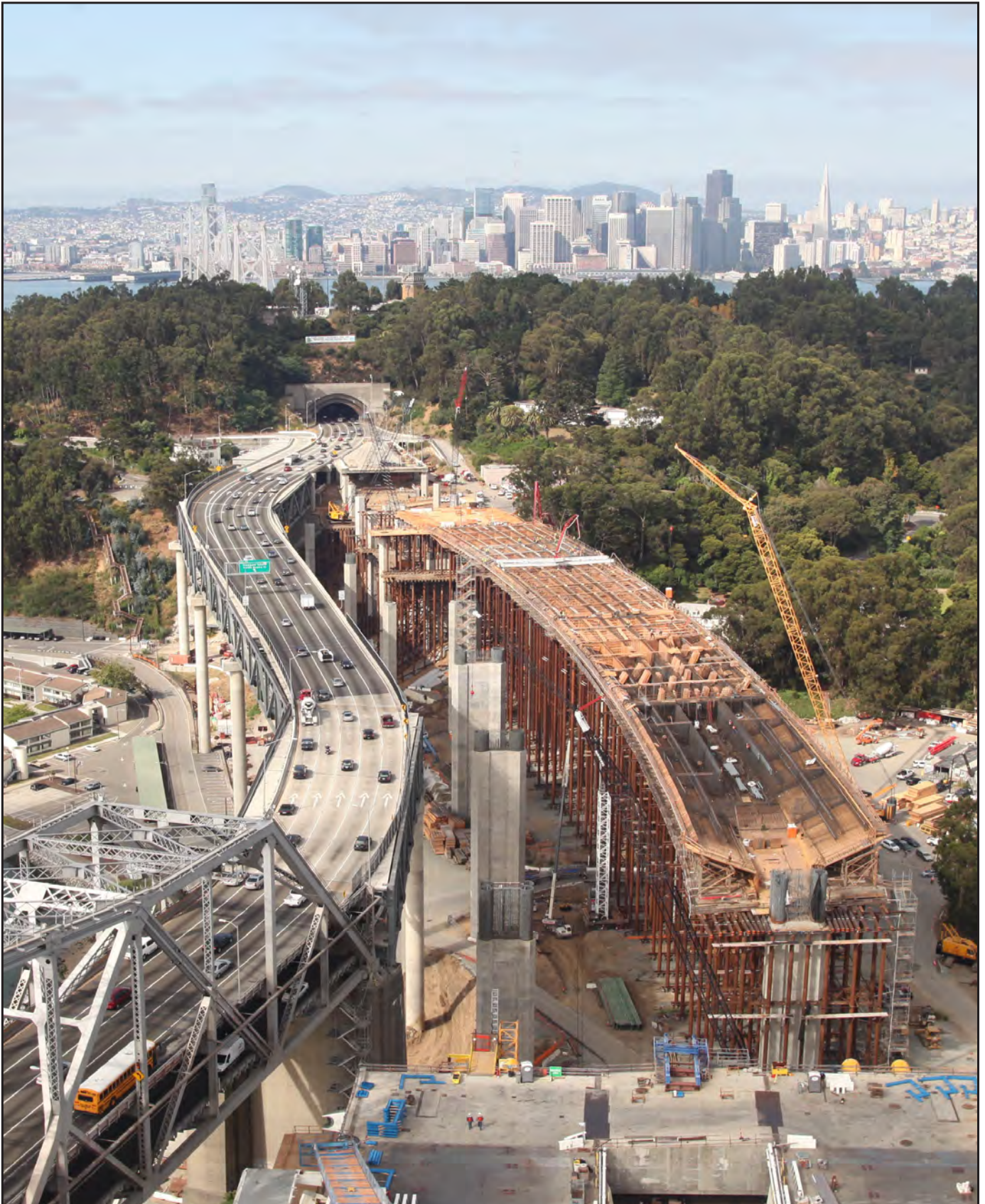
View from the top of the Self-Anchored Suspension Bridge's Tower Looking Down on the Yerba Buena Island Transition Structures #1 Westbound Falsework, Formwork and Rebar Installation in Progress
