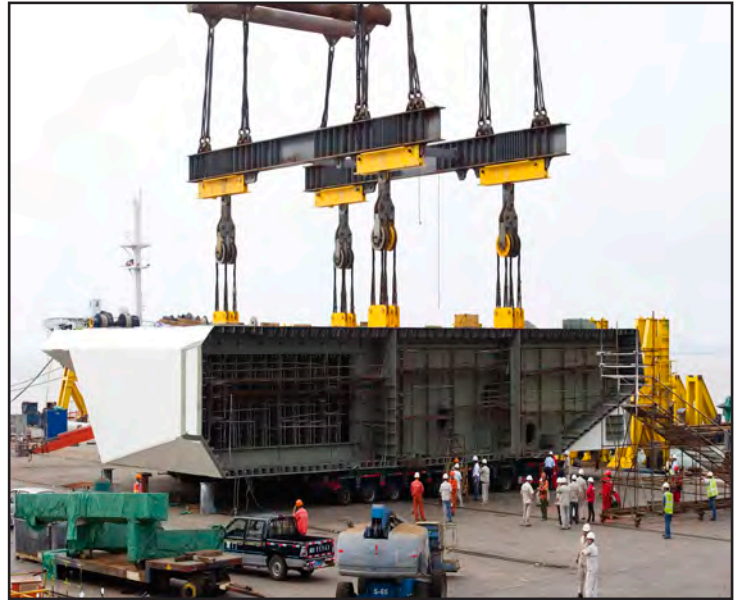
Loading Roadway Box 14 West onto the Ship - the Last Steel Segment Voyage
