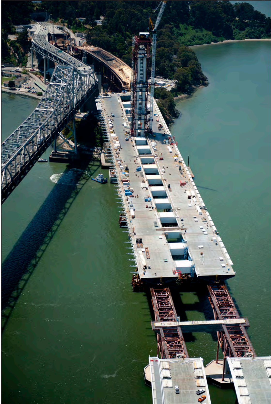
The Tower Saddle Being Installed atop the Tower of the Self-Anchored Suspension Bridge
