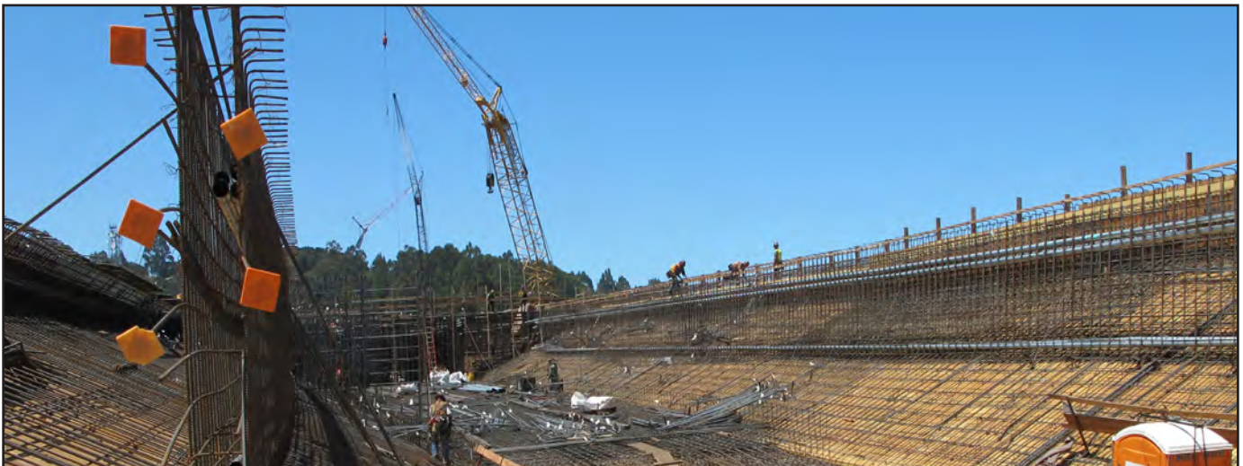
Yerba Buena Island Transition Structures #1 Westbound Falsework, Formwork and Rebar Installation in Progress
