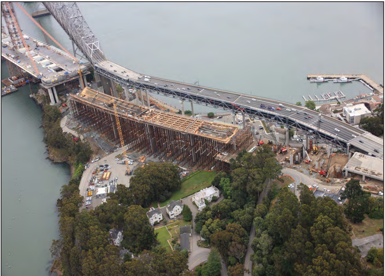
Aerial View of the Westbound Yerba Buena Island Transition Structure alongside the Existing Detour
