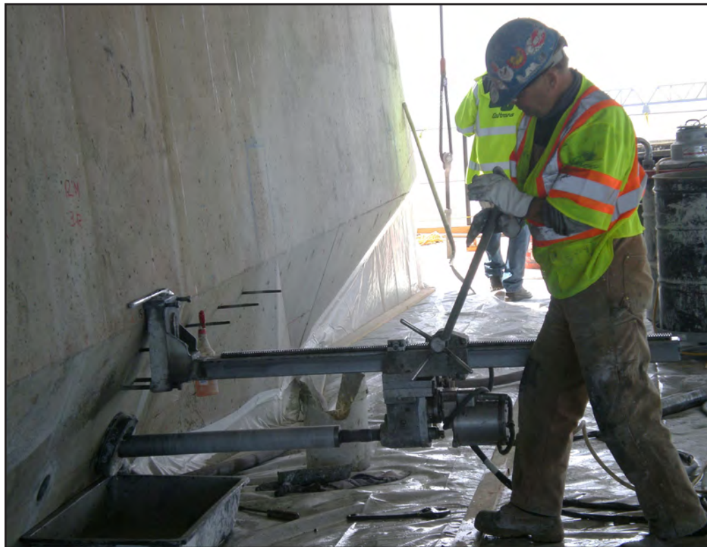
Core Drilling Operation Will Allow for Reinforcing Steel to Anchor into the Existing Bent Cap
