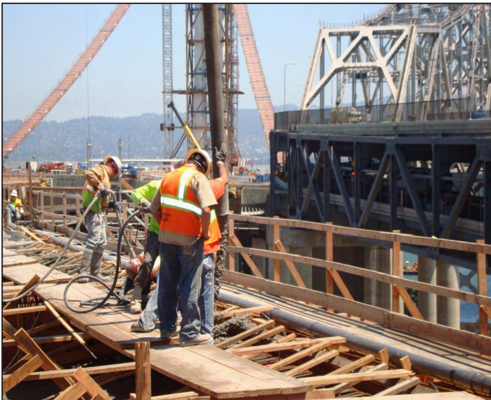
Yerba Buena Island Transition Structures #1 Westbound Concrete Pour with Newly Installed Catwalks to Tower in Background
