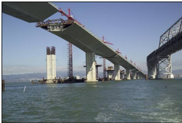
The Eastbound Roadway Section is to the left of the existing East Span (Looking East) 1.
