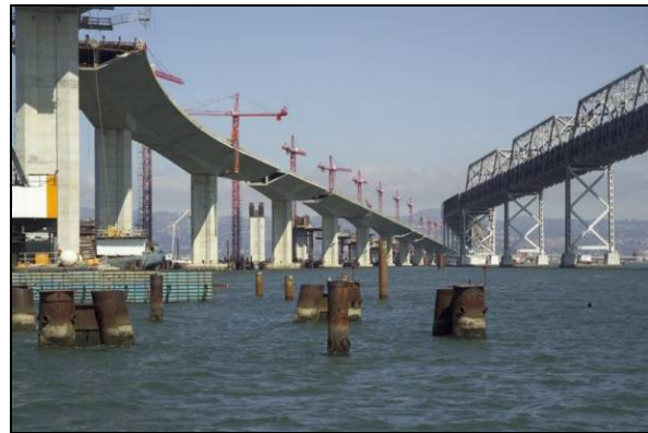
The Eastbound Roadway Section is to the left of the existing East Span (Looking East) 2.
