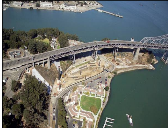
Aerial View of Pier Footing and Column Construction for the South-South Detour at YBI.
