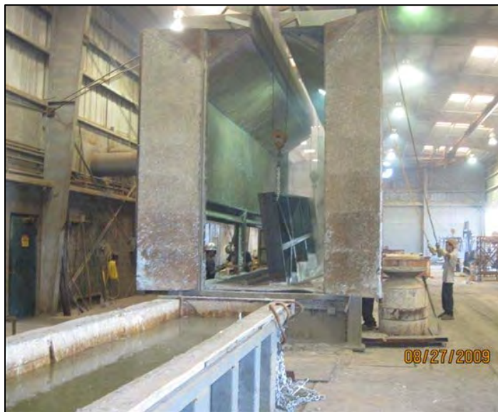
SAS Service Platform Upper-Frame Galvanizing, California
