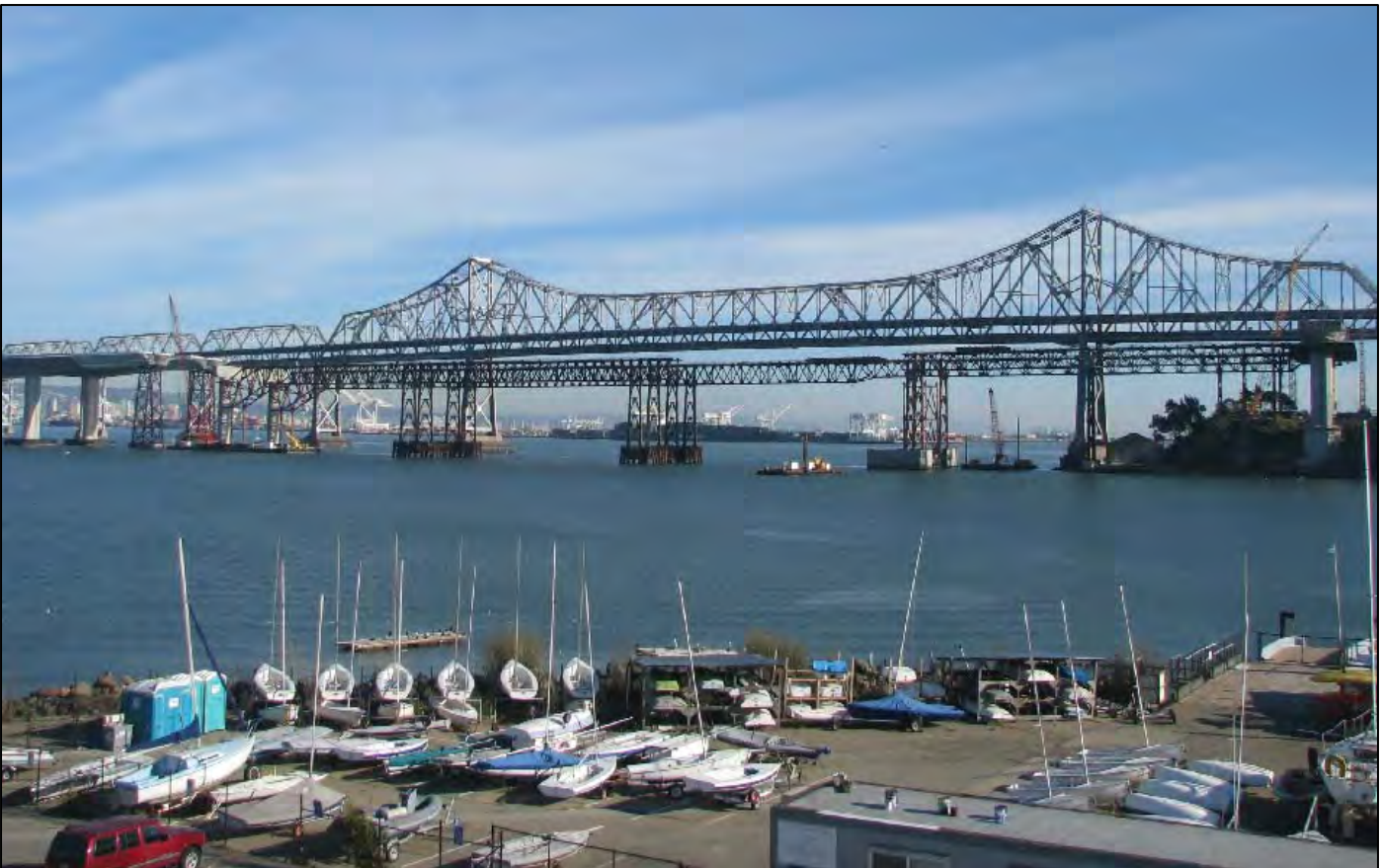
SAS Temporary Support Structures and Tower Erection Temporary Framing and the End of the completed Skyway on the Left
