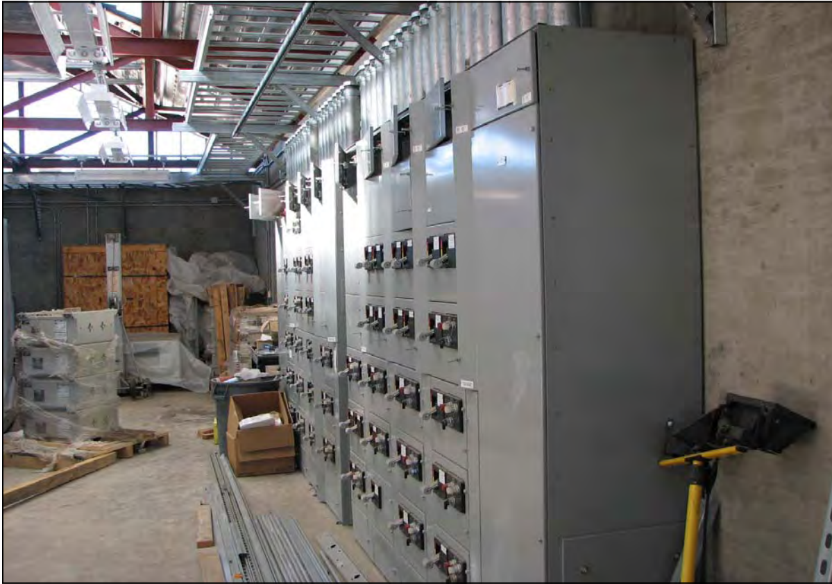
Oakland Touchdown Mole Substation Electrical Equipment
