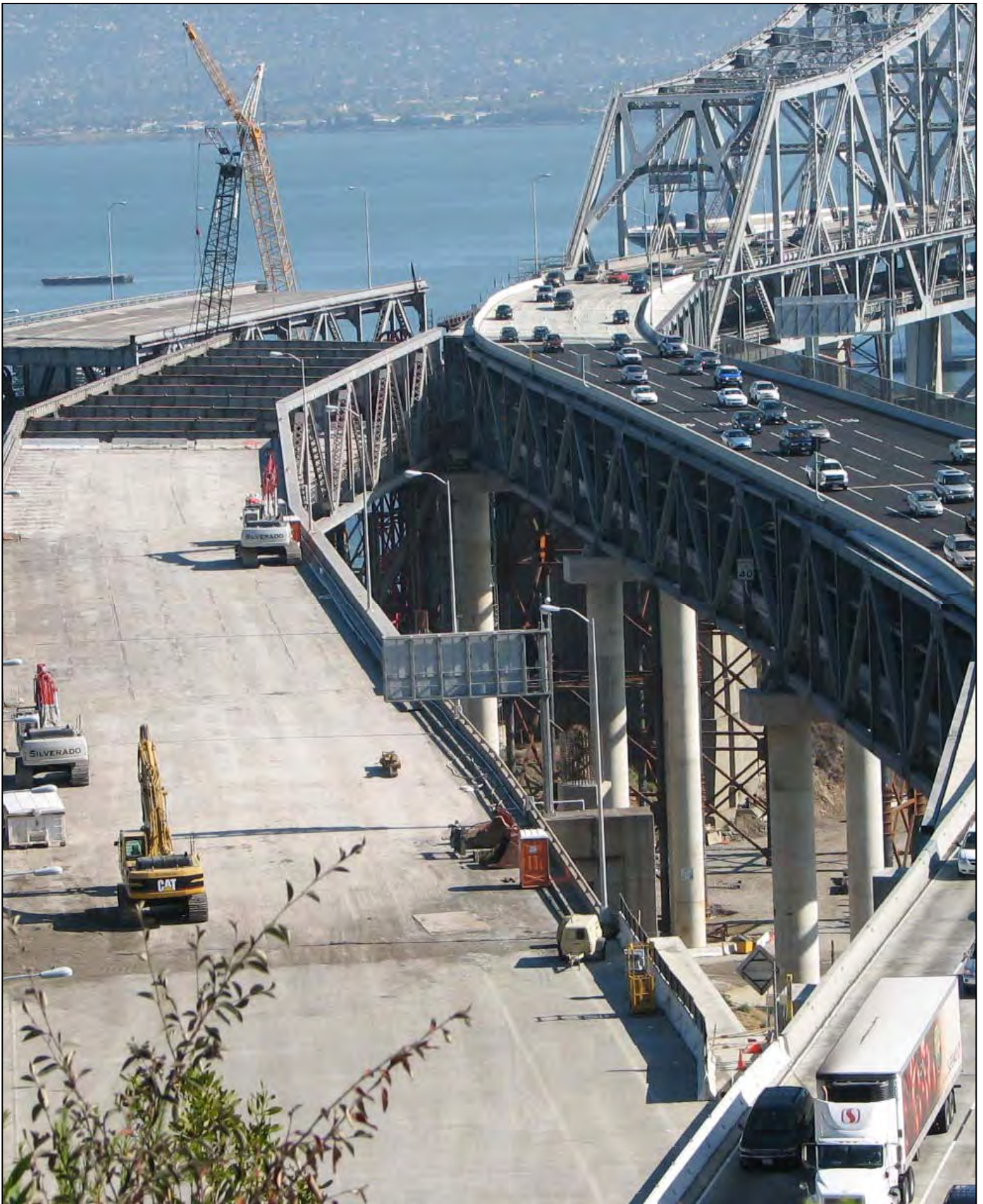
Existing Viaduct Bridge Spans YB3 & YB2 to the Left and the Detour Structure
