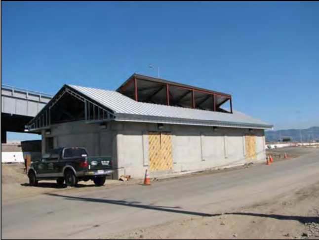
Oakland Touchdown Mole Substation
