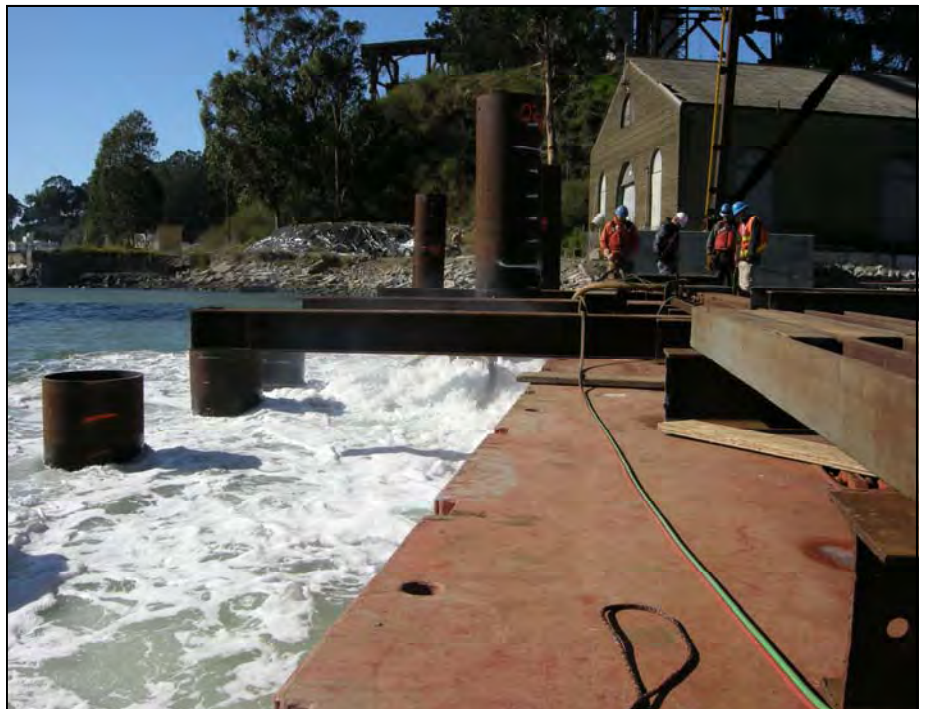
SFO Bay Bridge Air Bubble Curtain Sound Attenuation System (photo courtesy of Rob Aramayo)
