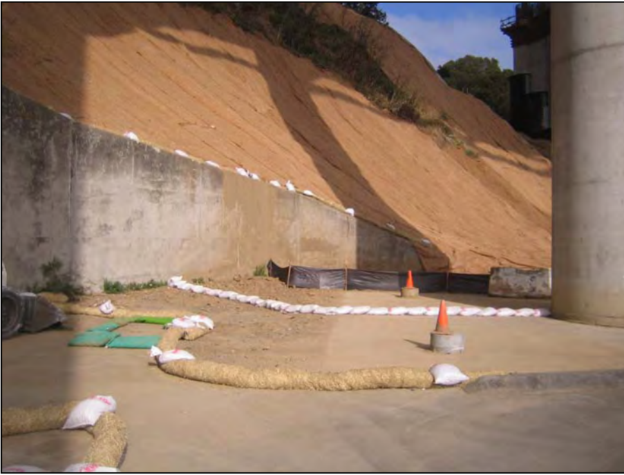
Yerba Buena Island Transition Erosion Control Matting, Silt Fencing, Fiber Rolls and Check Dams
