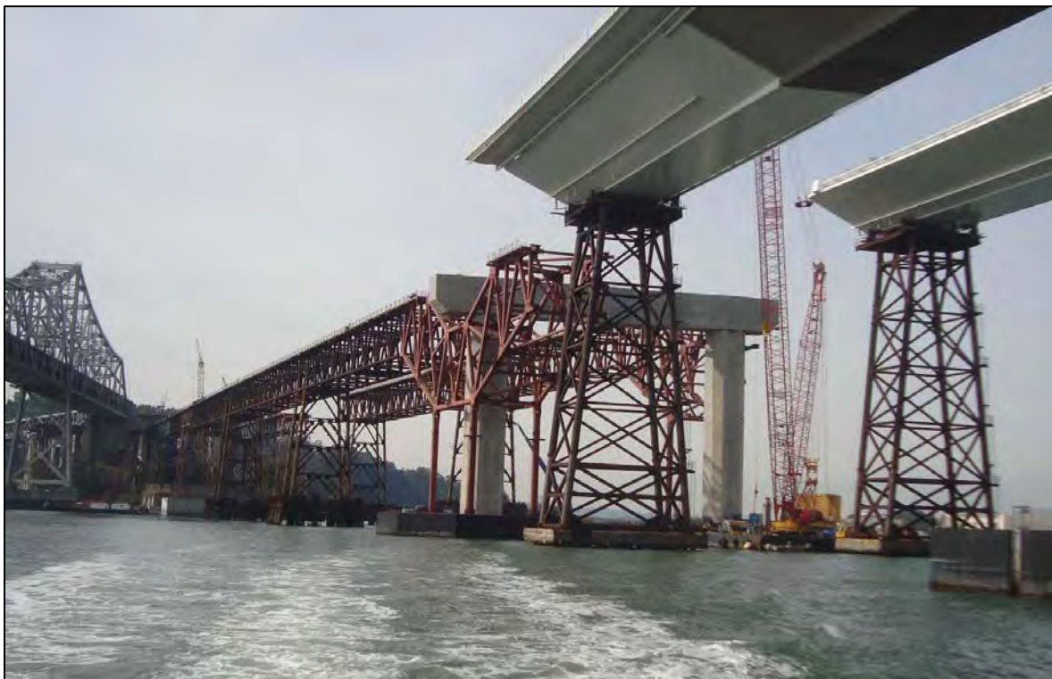
SAS - View from Temporary Support Structures East of H (E2) underneath Skyway
