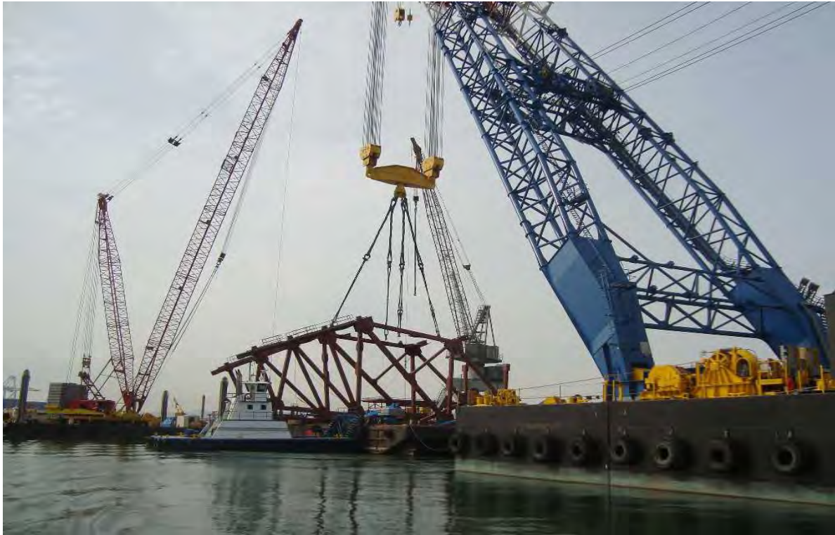
SAS - Pier 7 - Temporary Support Structures "W" D to E (Gap for Tower Erection)
