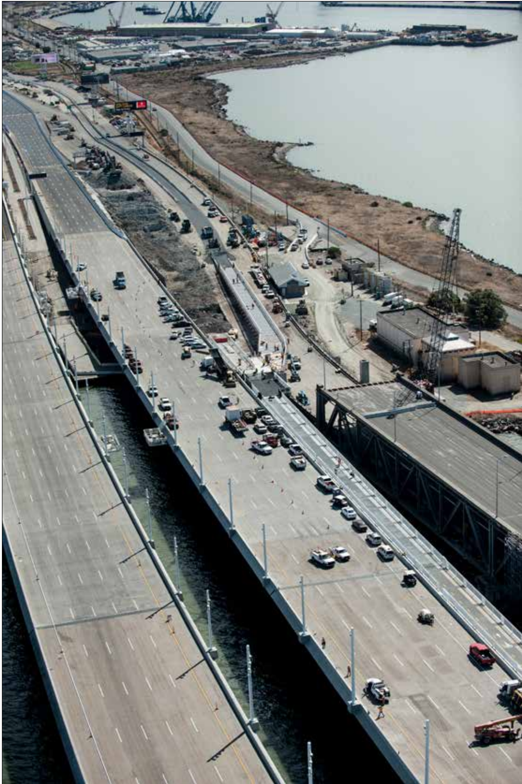
OTD Permanent Bike Path in Progress Looking east toward Oakland and Temporary Bike Path in Use at right
