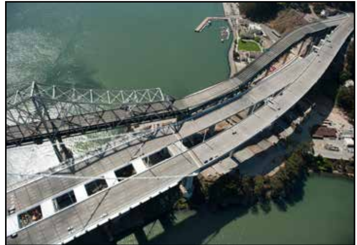
Cantilever section of the Old eastbound Bridge Section Included in the YBITS #2 Contract for Removal next to the New Bridge
