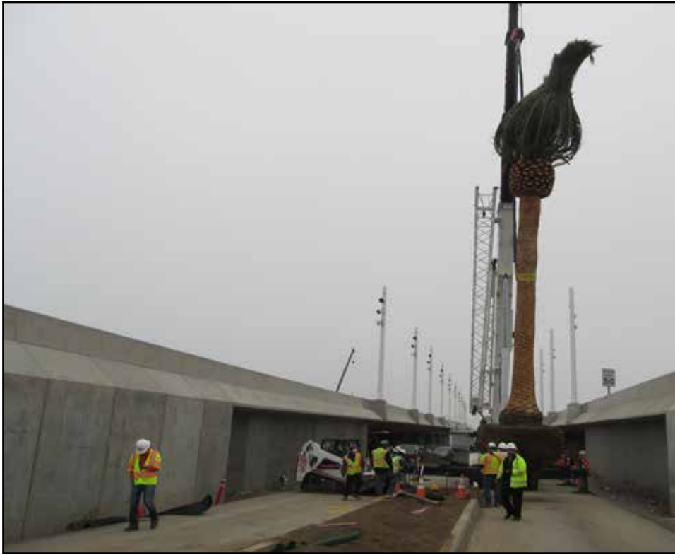
First Permanent Palm Tree Placement in Progress at OTD #2 between the New Bridge eastbound and westbound OTD Structures
