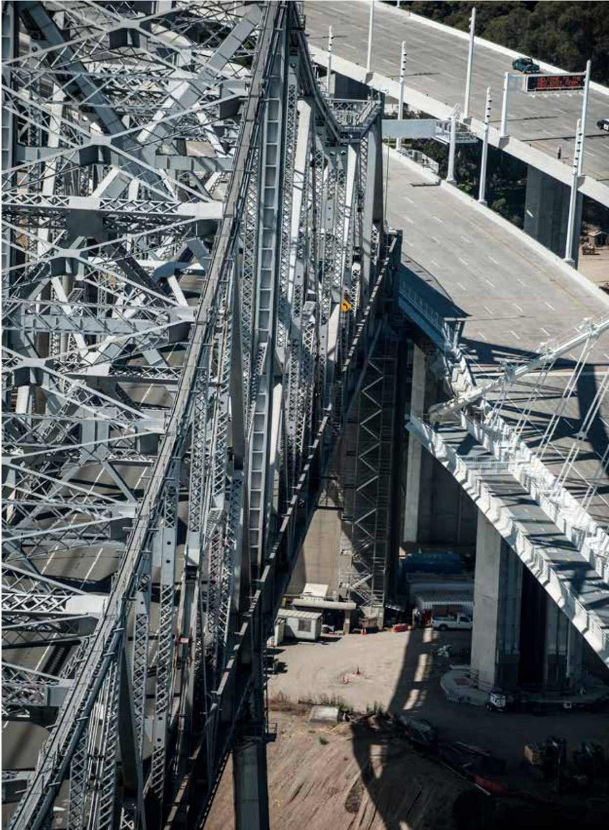
Permanent Structure at right and Cantilever of Old San Francisco-Oakland Bay Bridge Dismantling Underway at left
