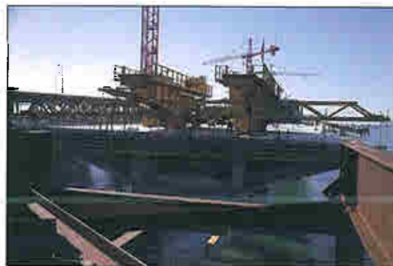
Use of Self Launching Erection Device (SLED) for Precast Concrete Deck Segments
