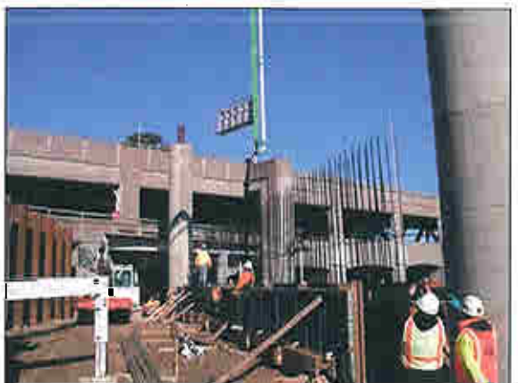
SoSoDet - Construction of Bent 48 grade beams along the former Southgate Road on Yerba Buena Island
