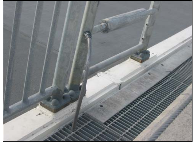
Skyway - Skyway Rail Bolt caps
